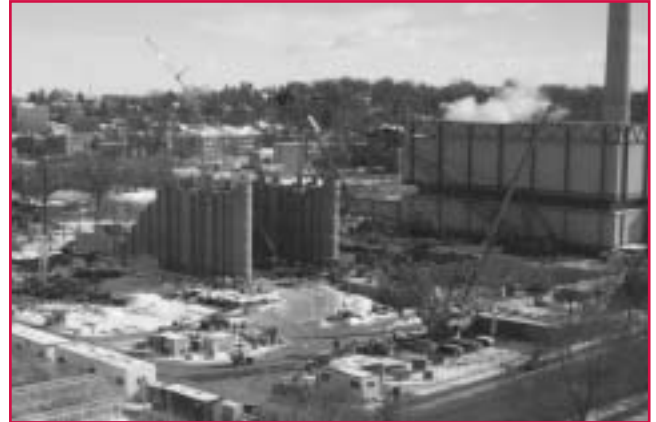
Contractors installed combustion and steam turbines plus steam generators in the first five months of construction on MGE's West Campus Cogeneration Facility. The site is located next to a UW heating and cooling plant.
